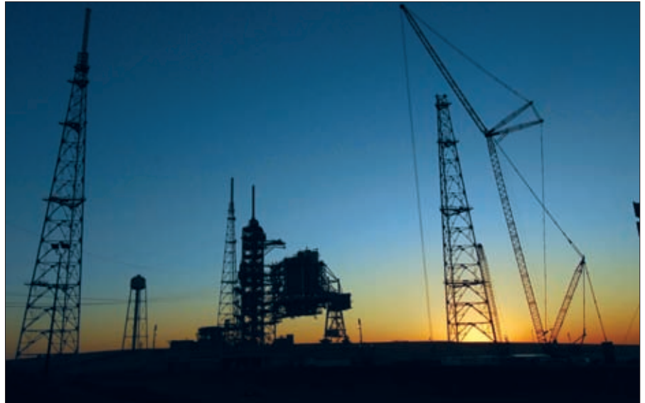
A February 2009 dawn reveals the newly erected lightning towers on Launch Pad 39B at KSC. The two towers at left contain the lightning mast on top; the one at right does not. At center are the fixed and rotating service structures that have served the space shuttle program. Each of the towers is 500 ft tall with an additional 100-ft fiberglass mast atop supporting a wire catenary system. (NASA)
