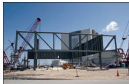
With the VAB as a backdrop, construction began in March at KSC on the new mobile launch platform for the Ares I booster.
